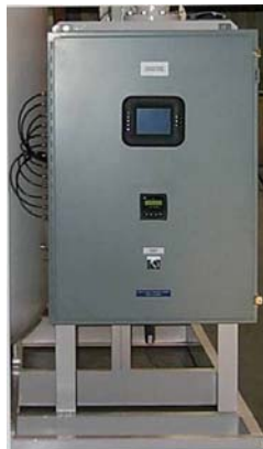
INSTRUMENT & CONTROLS PANEL
