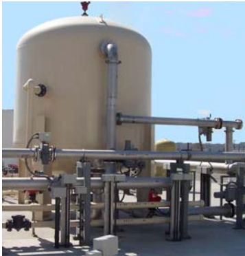
1100 GPM NITRATE REMOVAL SYSTEM
